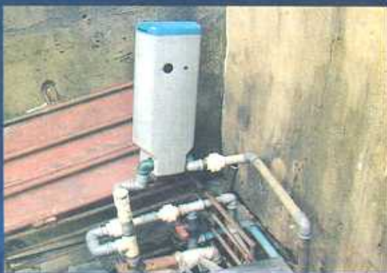
Meterbox on Customer Service Line
