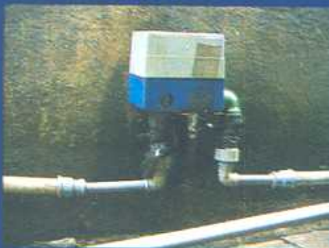
Meterbox on Customer Service Line
